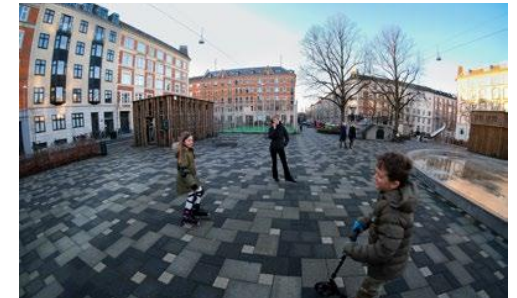
The top photo is a renovated public square in Frederiksberg, Denmark, called Langelands Plads, with Rockflow installed beneath it.
